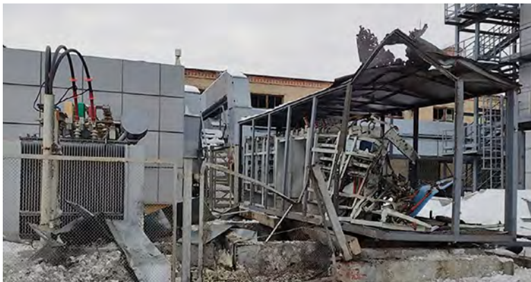
▲ A neutron source substation at Kharkiv Institute of Physics and Technology destroyed by Russian attacks on 6 March, 2022. © State Nuclear Regulatory Inspectorate of Ukraine.
