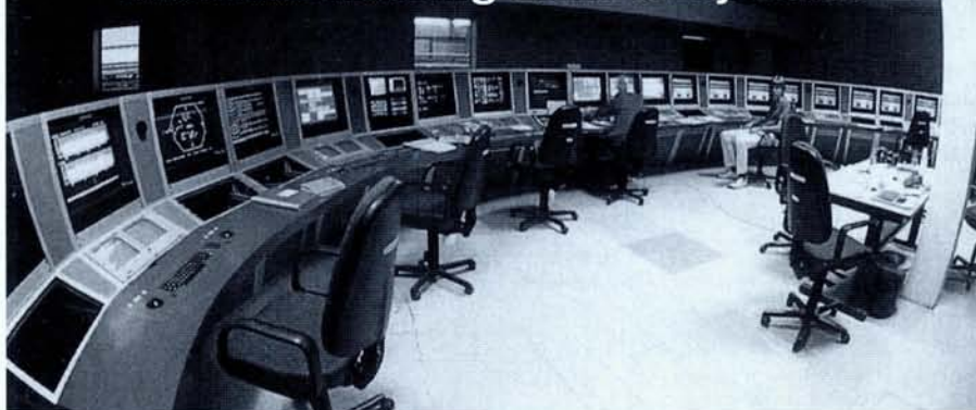
The control room of the HERA accelerator, DESY, Hamburg.
